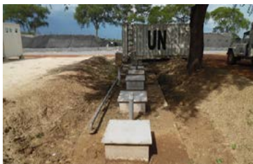
Waste water treatment
